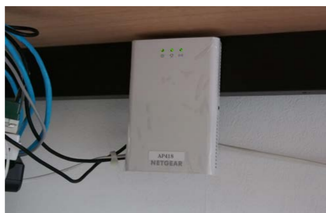
Access points were installed in guest rooms in inconspicuous places such as underneath furniture.
