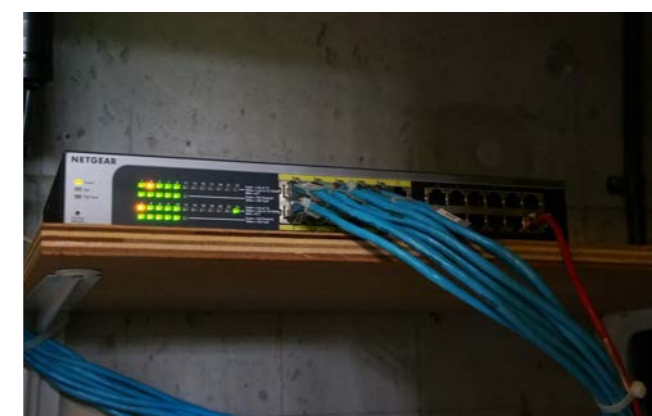
Floor switch (JGS524PE) installed behind the scenes on a guest floor. This switch powers the access points in all guest rooms on the floor via PoE.
